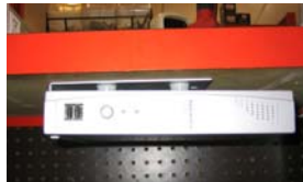
Thin Client installed in Bracket under counter.
